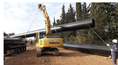
Figures 3 & 4: Safety aspects, e.g. attention is drawn when handling floating load on site
