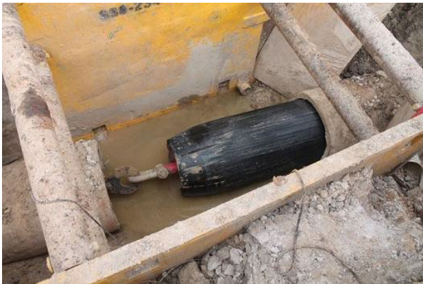
@PE100+ Association Picture: Close fit relining of old metal pipe with PE100-RC liner
