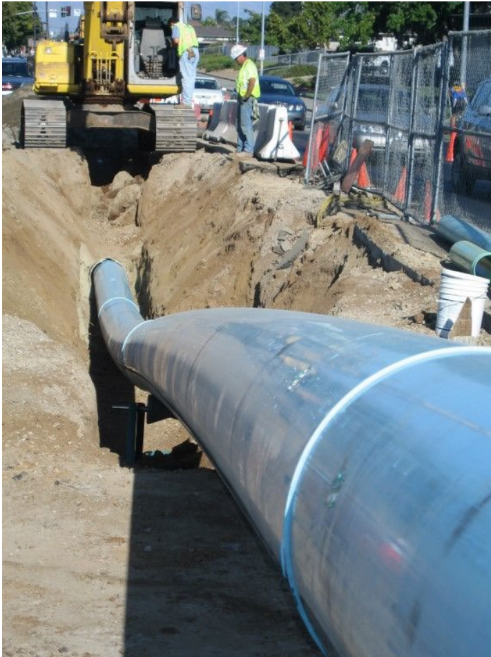
@PE100+ Association Picture: Slip lining of old media pipe with new PE100-RC pipe
